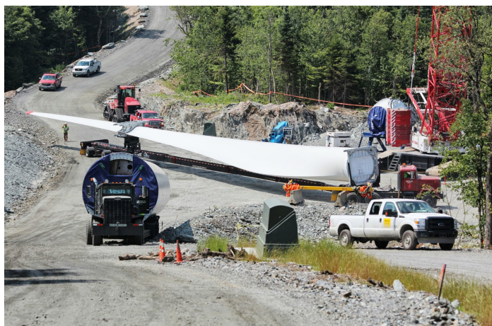
The exact location of the towers is determined after careful calculation of a number of factors. Coordinating the safe transportation of the turbines and towers and their placement at the site are key tasks for Vestas, Lone Star and Green Mountain Power.
